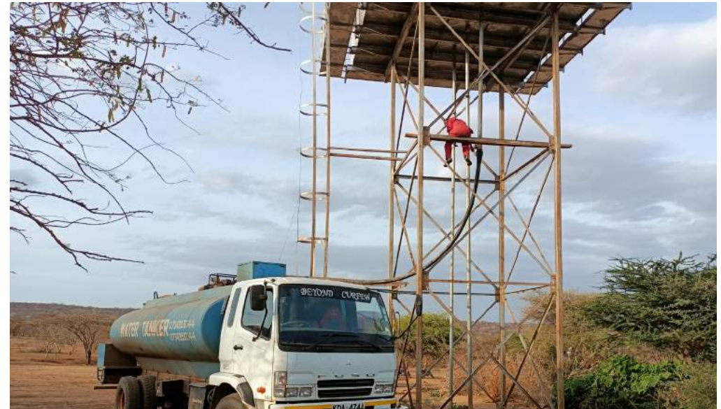
Filling up the water tank at Kamboe water point
